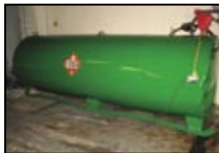
1,000-Gallon Diesel Tank
