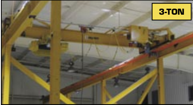
Free-Standing Bridge Crane
