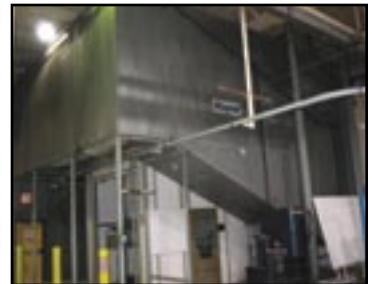
Rapid Conveyor to Ovens
