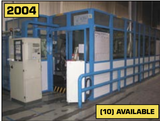
Grinding Cell Enclosure
