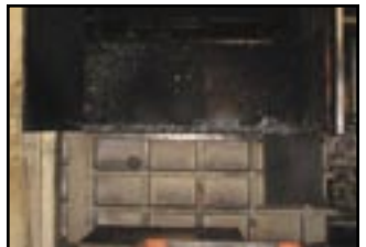
5' x 10' x 30" Melt Furnace
