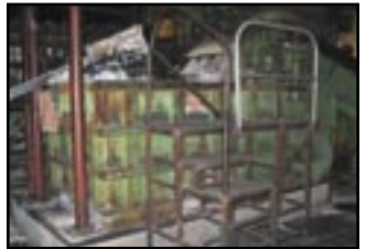
41" x 58" x 39" Melt Furnace
