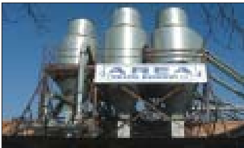
VIEW OF CYLCONE SYSTEM
