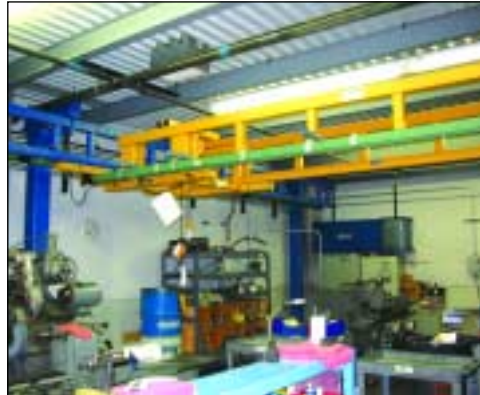
2-TON GORBELT FREE STANDING BRIDGE CRANE
