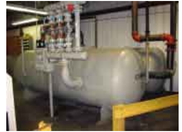
1,000 Gallon Compressed Air Reservoir System
