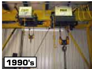
1990's 15,000 LB A-Frame Bridge Crane System
