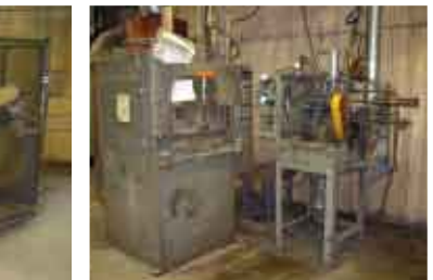
1984 Progressive Blasting System
