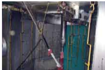
View of Inside Spray Booth
