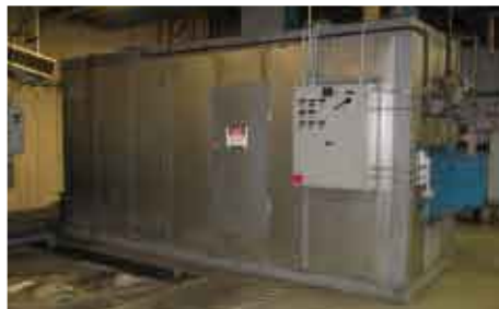
Gas Fired Dry Off Oven
