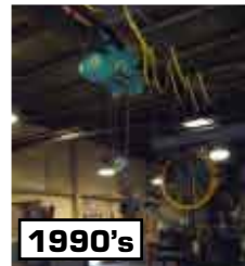
1990's 3-Ton P&H Over Head Bridge Crane
