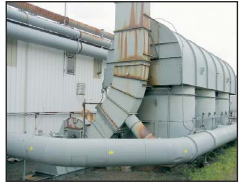
View of REECO 20,000 CFM fume oxidizer incinerator
