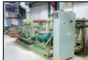
View of Air Compressor
