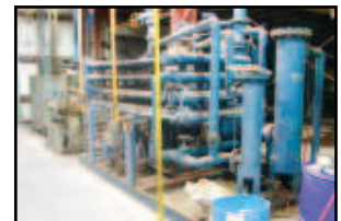
View of Air Compressor
