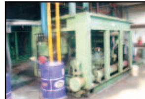
View of Air Compressor
