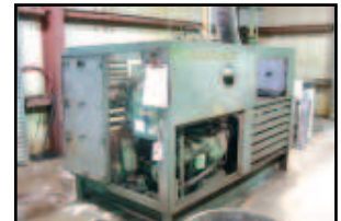
View of Air Compressor
