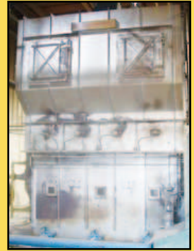
Gudgeon Thermal Reclamation System
