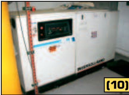
Ingersoll Rand Air Compressor
