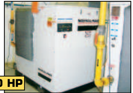
Ingersoll Rand Air Compressor
