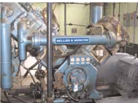
(2) Belliss & Morcom Air Compressors (NEW in 2001 & 1999)
