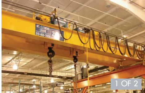
1 OF 2 MT. CLEMENS CRANE 20-TON DOUBLE-GIRDER BRIDGE CRANE; 35' SPAN
