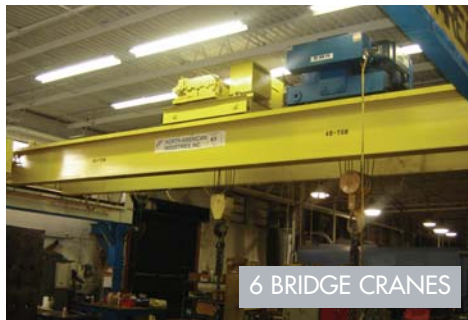
6 BRIDGE CRANES 40 TON BRIDGE CRANE
