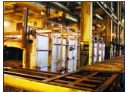
75' SURFACE COMBUSTION PUSHER FURNACE
