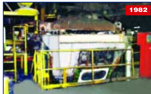
65 TON BBC VERTICAL CHANNEL HOLDING FURNACE MDL. IRV-11
