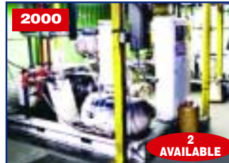
2000 GARDNER DENVER WATER COOLED AIR COMPRESSOR MDL. EBQQOC
