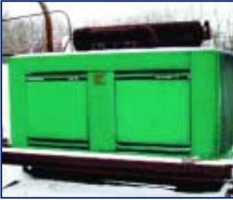
ONAN 180 KW STANDBY GENERATOR MDL. 180-ODFE-15R/2080IL
