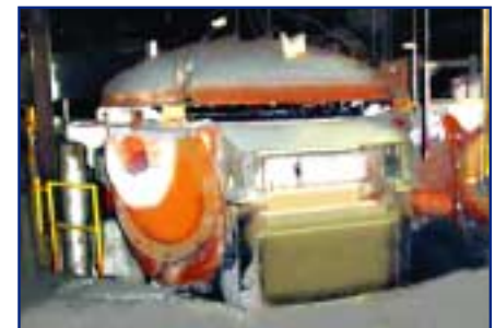
35 TON BBC VERTICAL CHANNEL HOLDING FURNACE MDL. IRV-8
