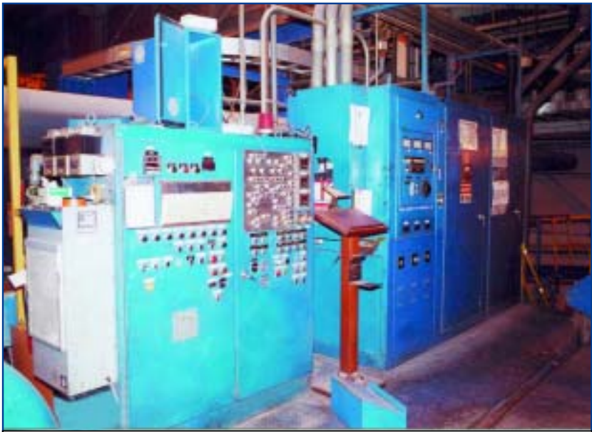
Offline Rebuild & Sintering Station w/300KW Power Supply
