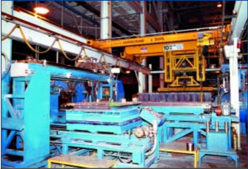
Hydraulic Mold Car & 10-T P&H Pick & Place Transfer Unit
