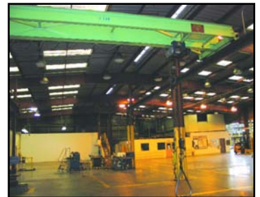
2-TON CM ELECTRIC HOIST CRANE
