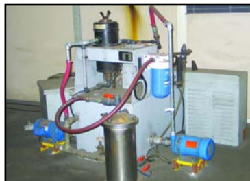
AGIE OIL PUMP STATION, MDL. DA-10
