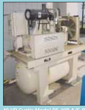
40 HP Curtis Model RS-40B A/E-B 160 Air Cooled Rotary Screw Horizontal Tank Mounted Air Compressor
