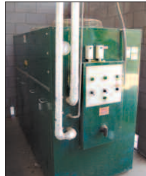
SCHREIBER WATER CHILLER
