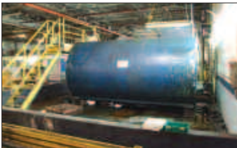
FLUID STORAGE SYSTEM
