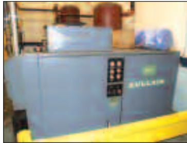
75 HP SULLAIR ROTARY SCREW AIR COMPRESSOR
