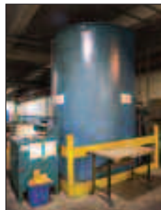
DEIONIZING WATER SYSTEM
