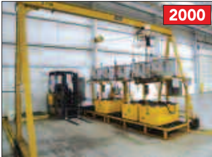
2000 BATTERY CHARGER SYSTEM W/MATERIAL HANDLING
