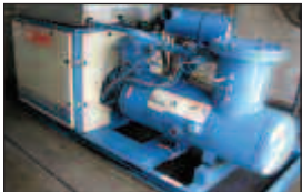
50 HP QUINCY AIR COMPRESSOR
