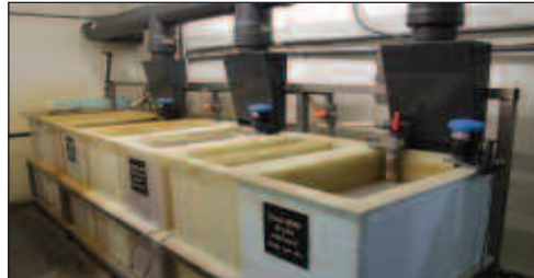
ANO-ETECH CLEANING LINE
