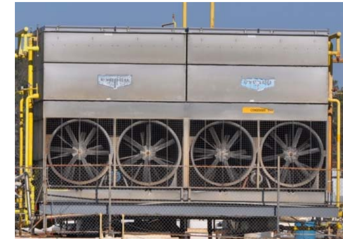
(5) Evapco & Frick Evaporative Condensers
