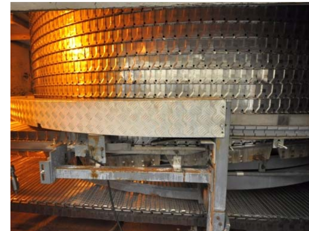
(6) Frigoscandia & York Ammonia Spiral Freezers
