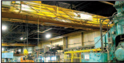
ASSORTED BRIDGE CRANES
