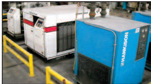
AIR COMPRESSOR SYSTEM & DRYER
