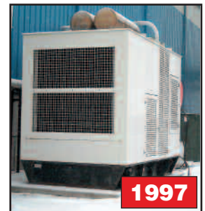
ONAN STANDBY DIESEL GENERATOR
