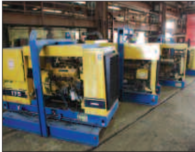
CATERPILLAR DIESEL GENERATOR SET
