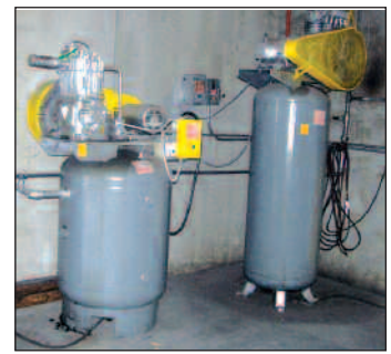
VIEW OF AIR COMPRESSORS
