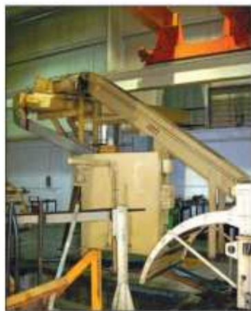
UNDERGROUND SCRAP REMOVAL SYSTEMS - BUILDING #3
