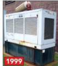
1999 DETROIT DIESEL SPECTRUM 100 GENERATOR
