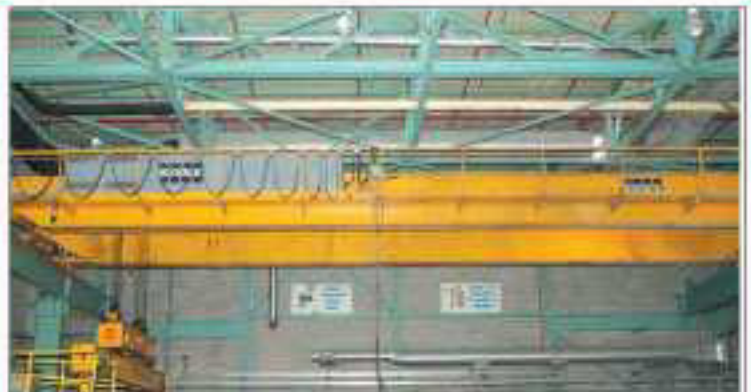
40 TON 20/20 KONE 8 WHEEL DOUBLE DROP OVERHEAD BRIDGE CRANE, S/N CI-4289, Total Cap. 40 Ton, Cap. Each Hoist 20 Tons, 77' 0" Span, 68' 0" Lift, Location: Appleton, WI
