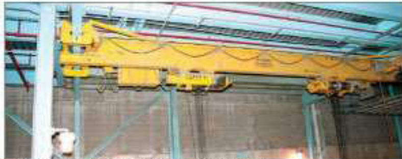
20 TON 11/10 WISCONSIN CRANE & HOIST OVERHEAD BRIDGE CRANE
