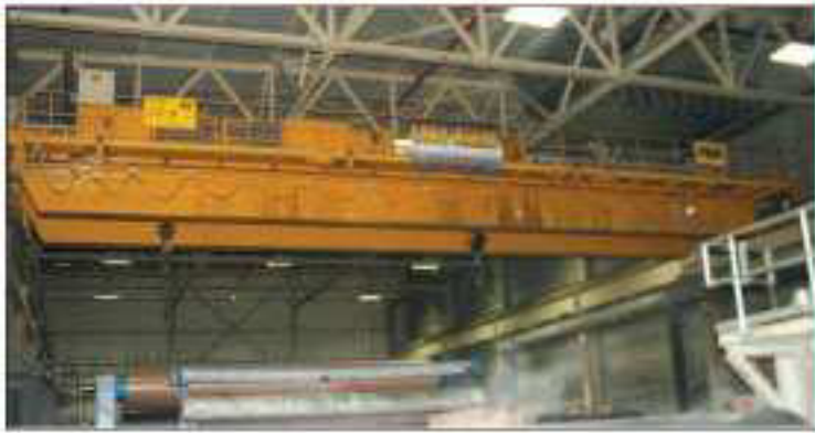
62 TON 31/31 P&H DUAL TROLLEY BRIDGE CRANE, S/N C27140, Cap. Each Trolley 31 Ton, Span 72', Lift Each Hoist 27' 5", Welded Box Girders, 5 Step Variable Speed, 105 Magnetorque Braking, Independent End Truck Drive, Radio Controlled
