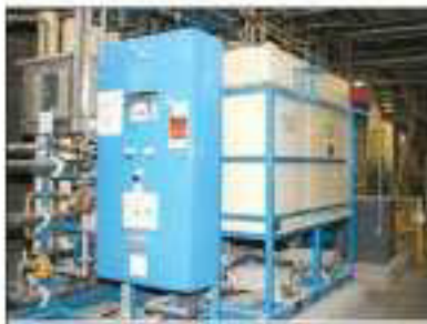
PALL CORP MDL. ARIASM WATER TREATMENT SYSTEM
