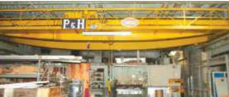
26 TON P&H DOUBLE GIRDER OVERHEAD BRIDGE CRANE
