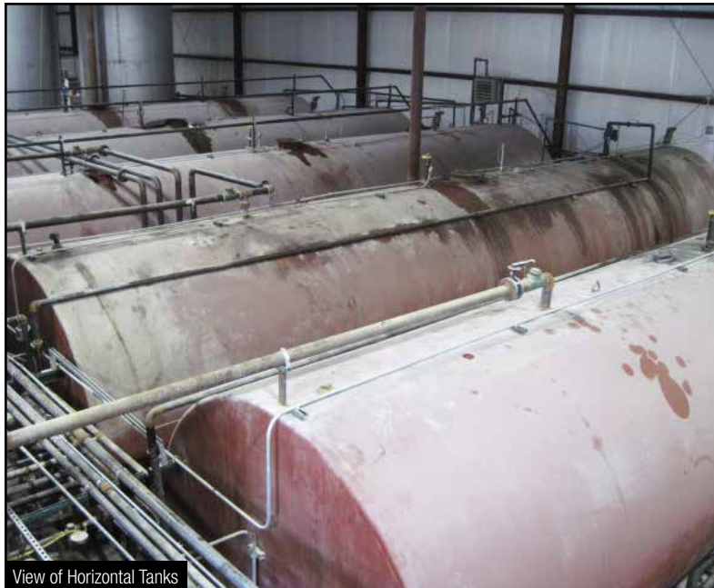
View of Horizontal Tanks
