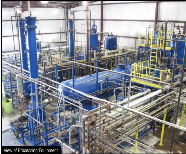
View of Processing Equipment
