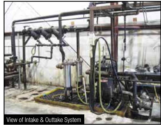
View of Intake & Outtake System
