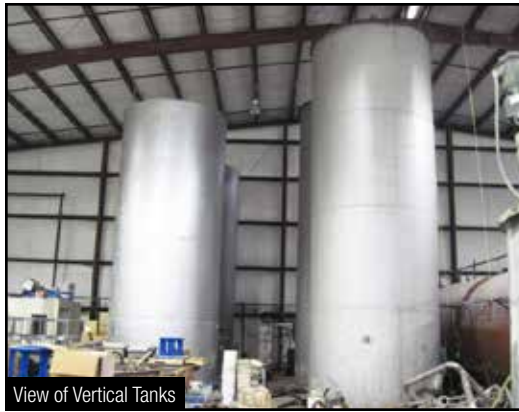
View of Vertical Tanks
