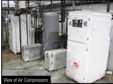
View of Air Compressors
