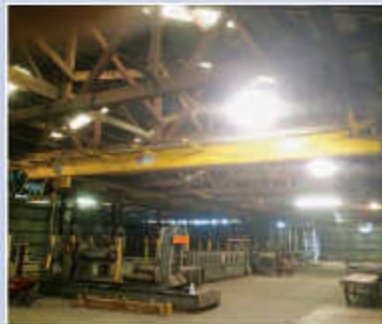
B&H 5 Ton Bridge Crane
