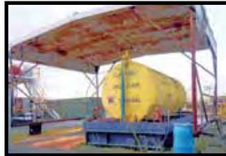
7,000 GAL. DIESEL STORAGE TANK STATION
