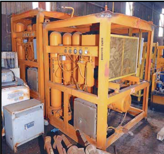
(2) HIGH PRESSURE RECIPROCATING AIR COMPRESSOR SYSTEMS
