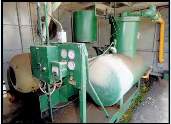
SULLAIR 300 HP ROTARY SCREW AIR COMPRESSOR
