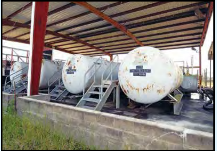
OIL STORAGE AND RECOVERY FACILITY
