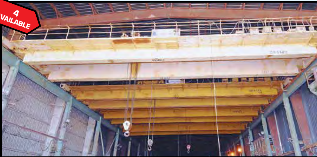
LANDEL 40 T. OVERHEAD BRIDGE CRANES
