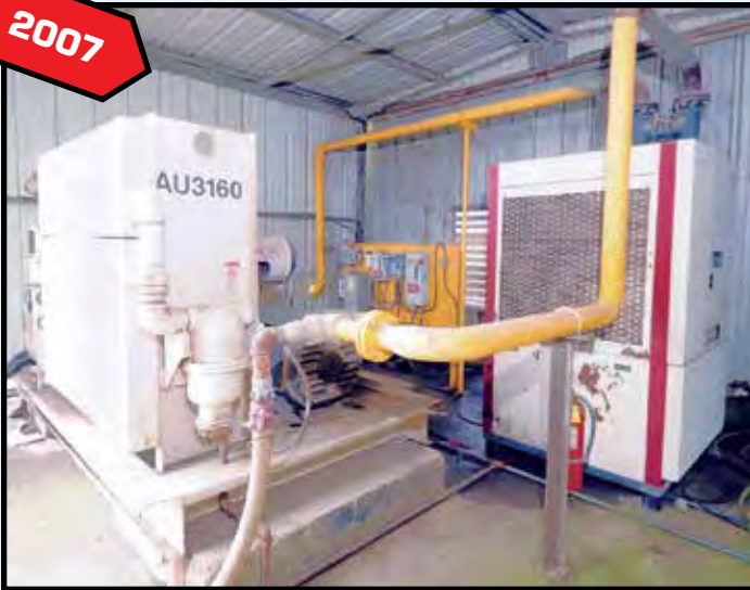
GARDNER DENVER 300 HP COMPRESSOR AND DRYER
