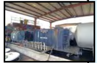
OIL STORAGE AND RECOVERY FACILITY
