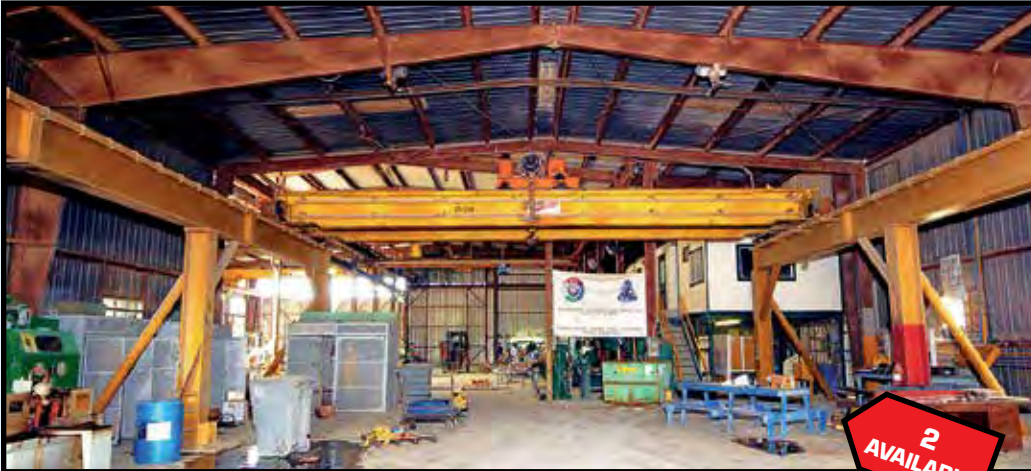
KRANCO 25 T. BRIDGE CRANES ON FREE-STANDING RUNWAY
