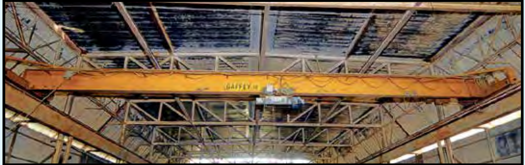
GAFFEY 10 T. SGL. GIRDER OVERHEAD BRIDGE CRANE
