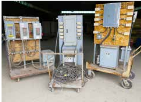
Assorted Electrical Panels
