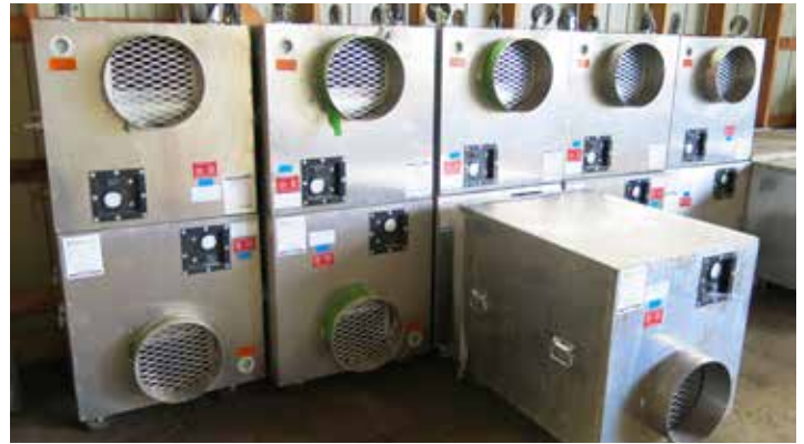
View of Air Changers
