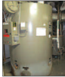
FULTON NAT. GAS BOILER
