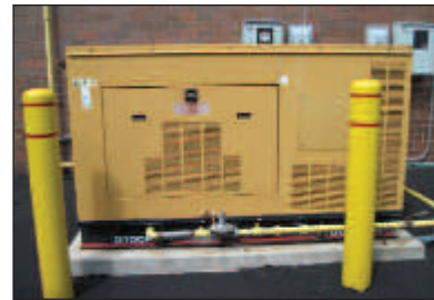
OLYMPIAN 100-KW EMERGENCY GENERATOR
