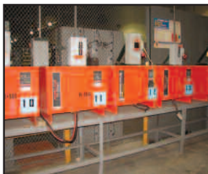
VIEW OF BATTERY CHARGERS
