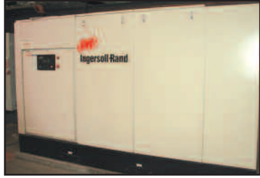
INGERSOLL RAND SSR 150HP COMPRESSOR
