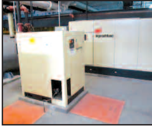
INGERSOLL RAND AIR COMPRESSORS
