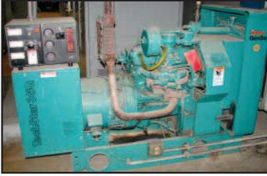
ONAN TELSTAR 35G NATURAL GAS GENERATOR
