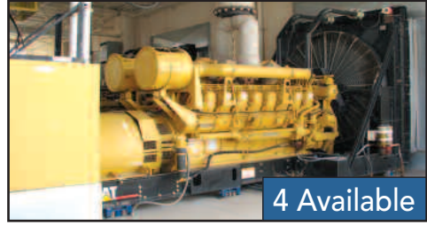
CAT 3516 DIESEL GENERATOR
