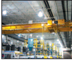
HOIST EQUIPMENT OVERHEAD CRANE
