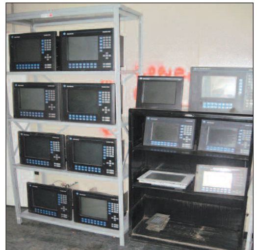
ALLEN BRADLEY PANELVIEWS, BOARDS AND CARDS
