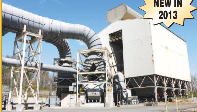
Schust Engineering Melt Shop Baghouse
