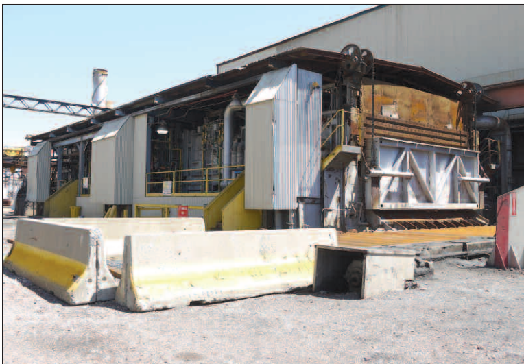
NATURAL GAS FIRED SLAB REHEAT FURNACE
