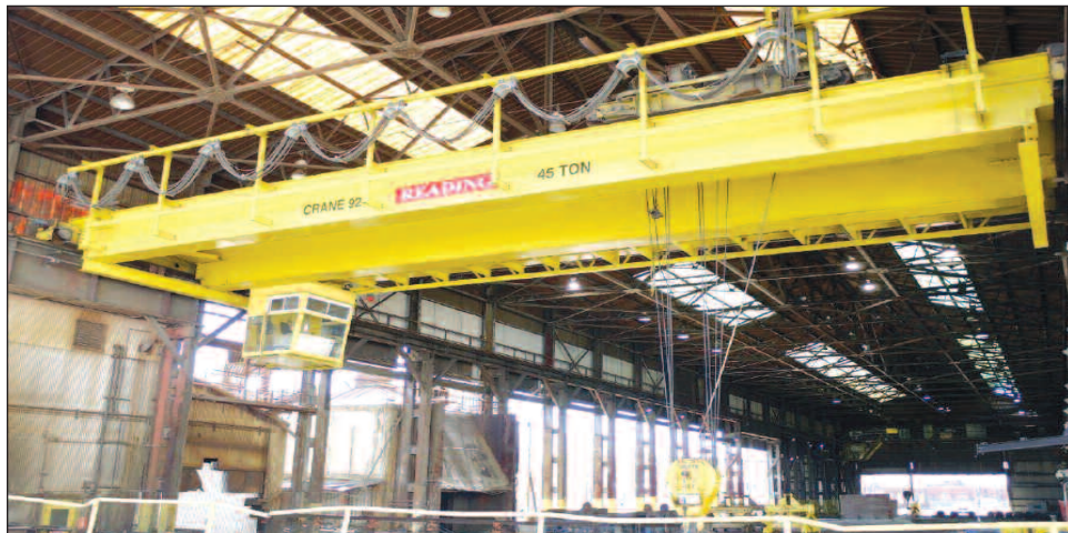
READING 45 TON OVERHEAD BRIDGE CRANE
