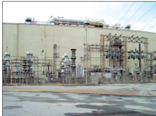
VIEW OF ELECTRICAL SUBSTATION
