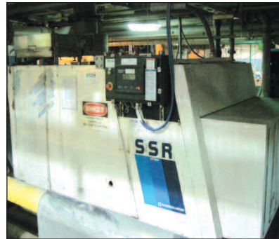
I.R. SSR XF250 Air Compressor
