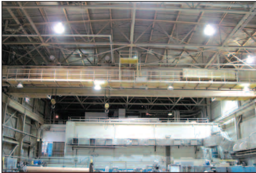
(2) Shepard Niles 70 Ton Bridge Cranes
