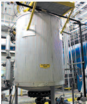
1,000 GAL. SS TANK
