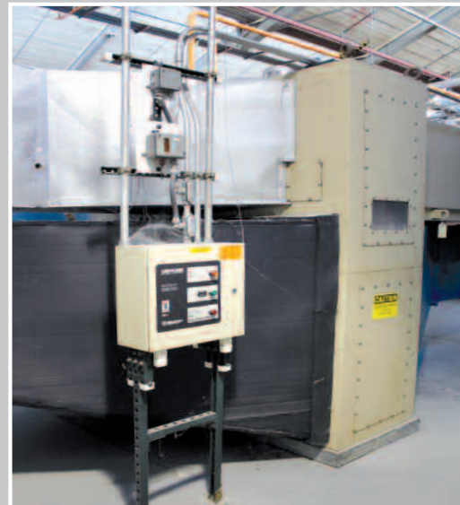
MUNTERS CARGOCAIRE DESICCANT AIR DRYER
