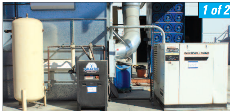
Ingersoll Rand 100 HP Air Compressor, w/Air Dryer & Air Receiving Tank
