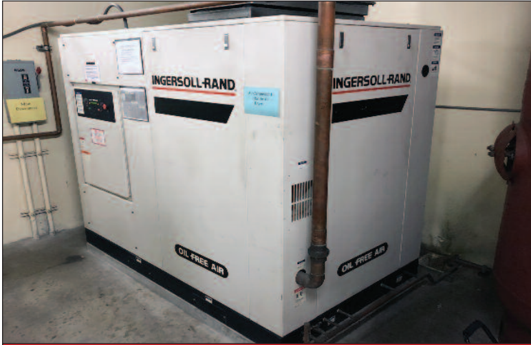
Ingersoll Rand Oil-Free 50 HP Air Compressor
