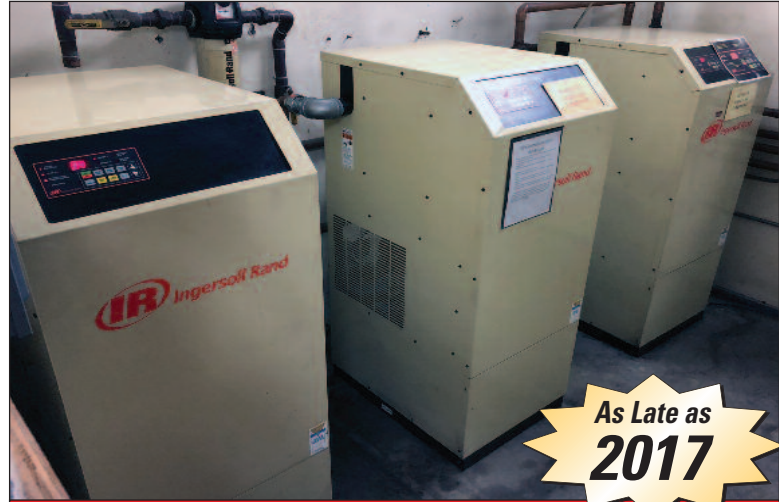
Ingersoll Rand Air Dryers
