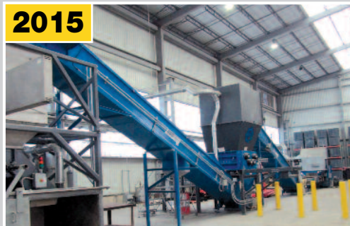
View of Shredding Line
