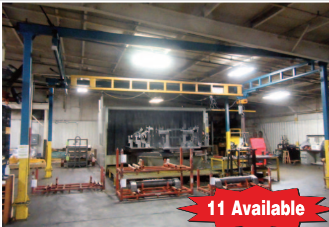
View of GORBEL Free Standing Bridge Cranes
