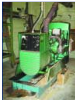
85 KW ONAN STAND BY GENERATOR, MDL. 8SKR
