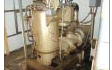
Quincy Rotary Screw Air Compressor
