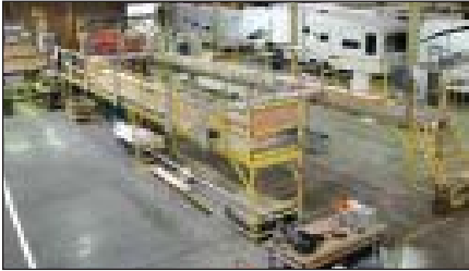
10' X 85' Fifth Wheel Assembly Scaffold System
